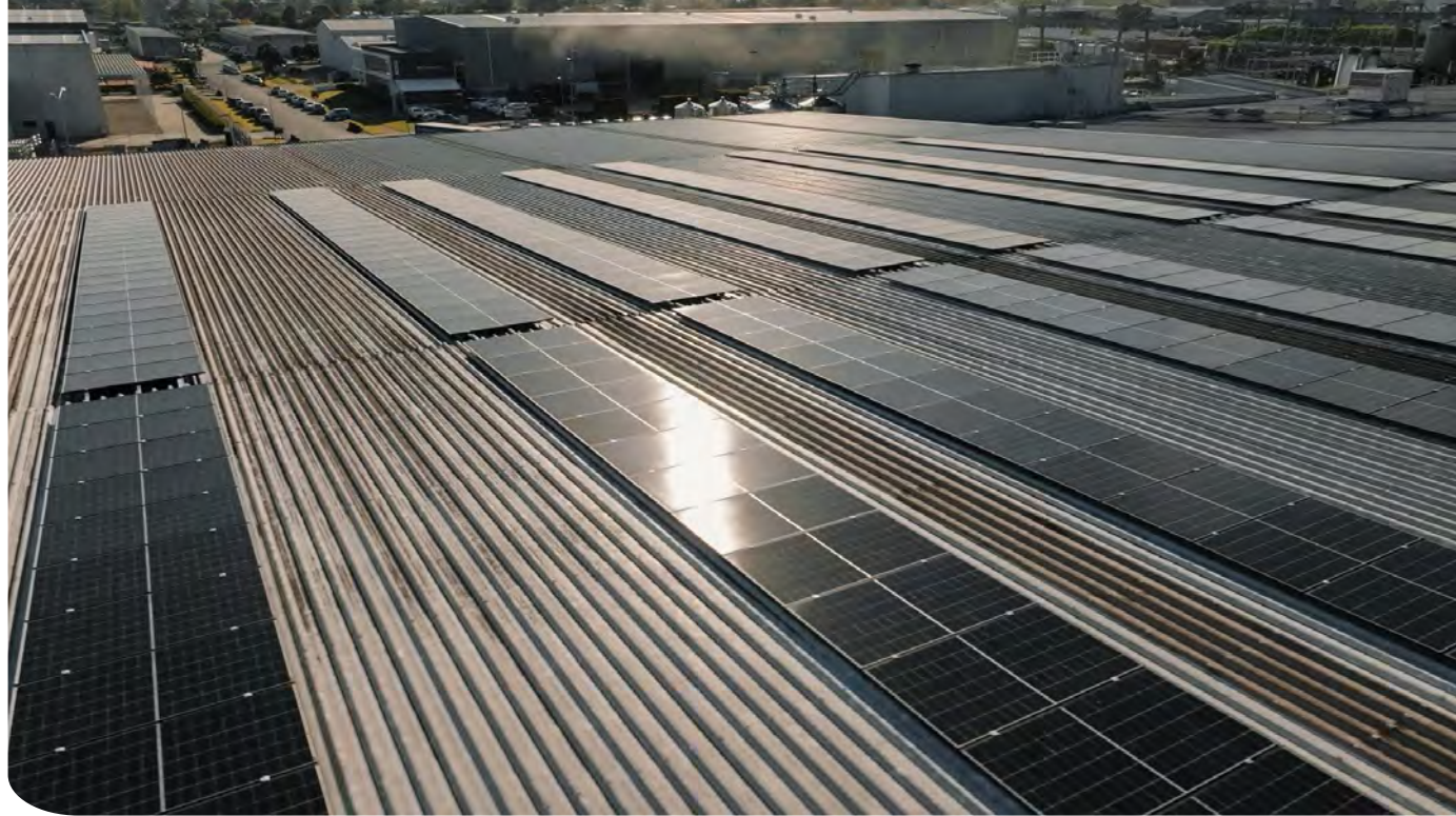
In partnership with Meridian, Lion NZ has installed one of the country's largest rooftop solar arrays in East Tamaki.
