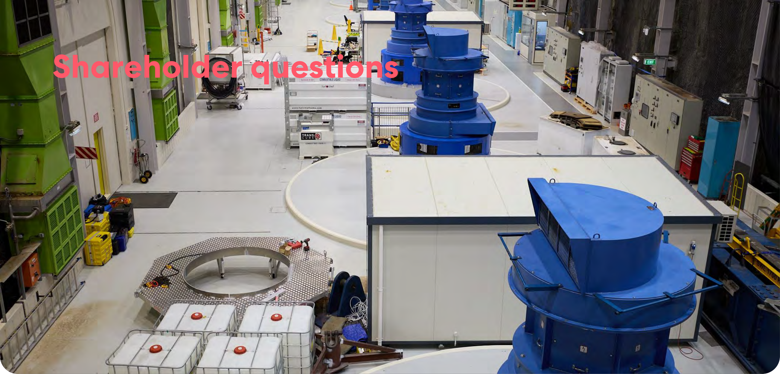
Manapouri Power Station in Fiordland.
