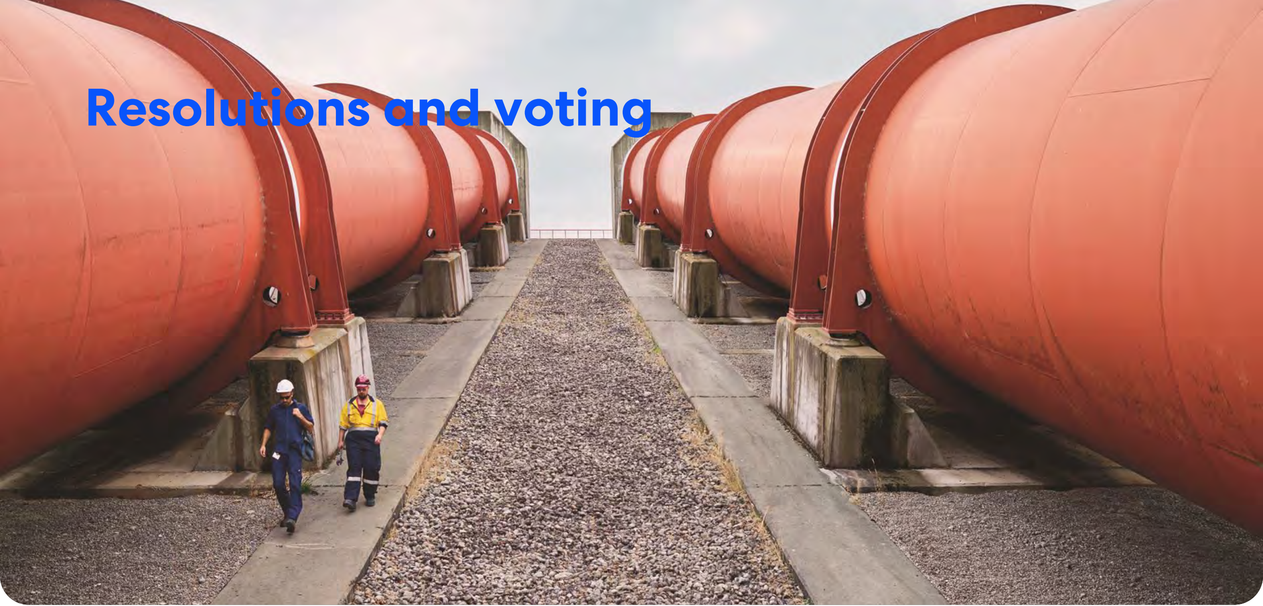
Ōhau A Power Station, South Canterbury.
