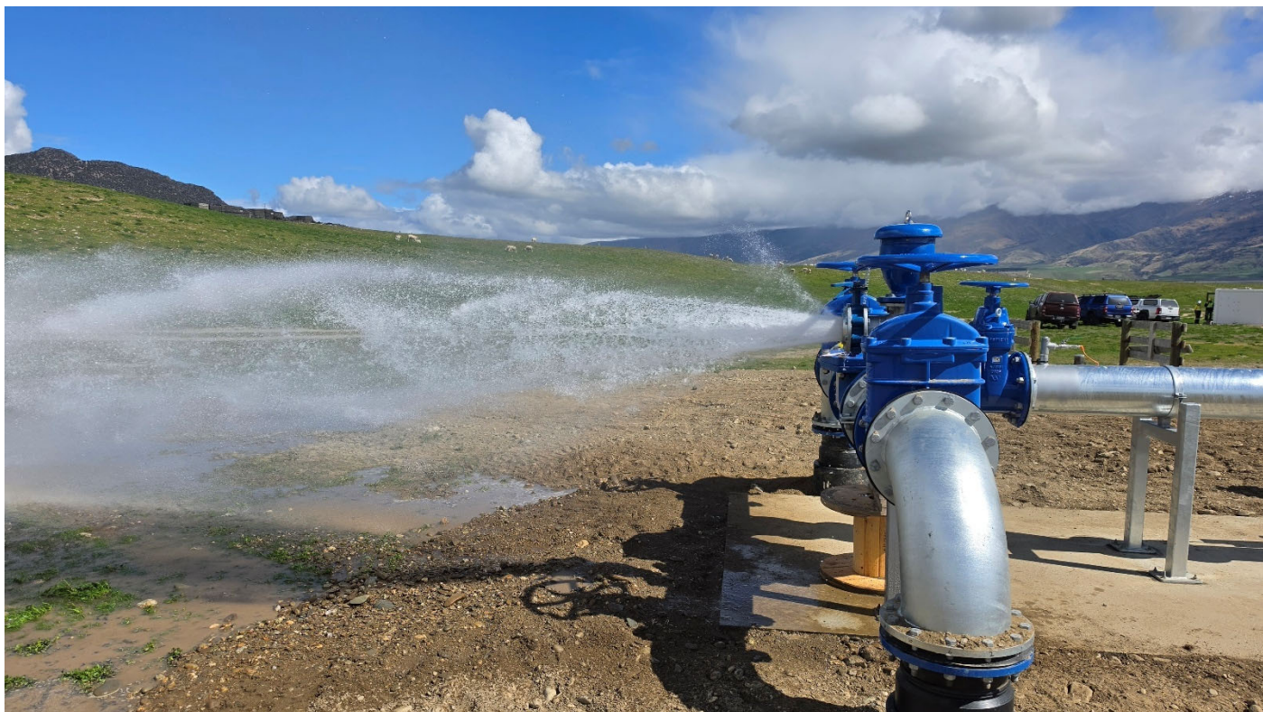
Figure 6. Successful commissioning test of the raw water pipeline manifold at Bendigo Aquifer bore.
