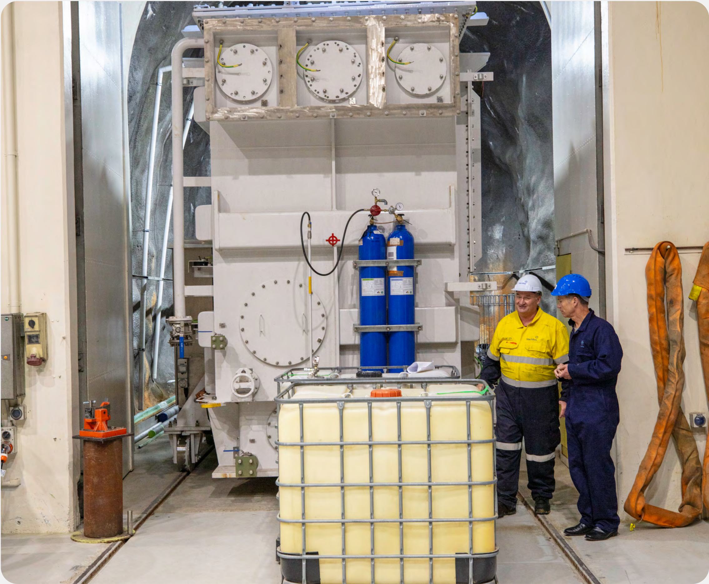
ABOVE: Transformer vault, Manapouri Power Station.
