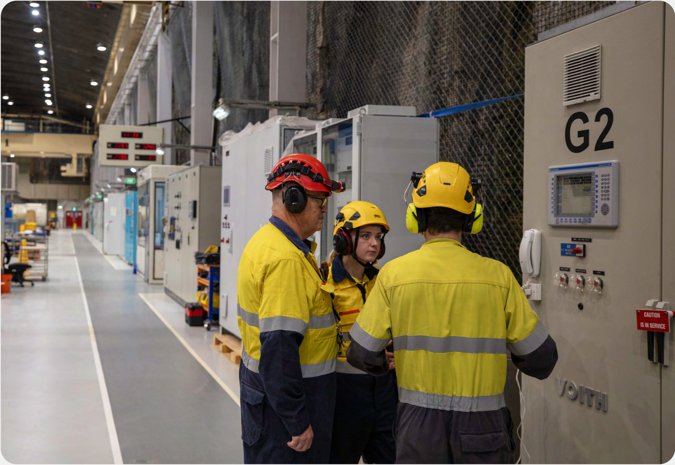
ABOVE: Manapouri Power Station, Fiordland.
