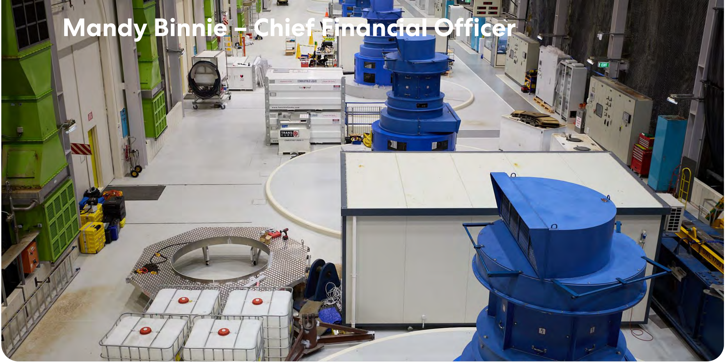
Meridian's Manapōuri hydro power station
