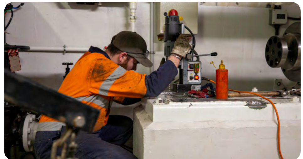
ABOVE: Benmore Power Station, Ōtematata.
