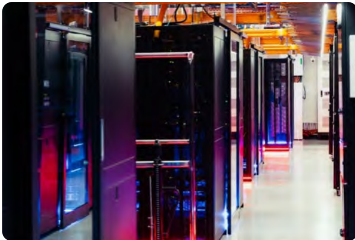
Datacentre220 – our first Express Connect installation
