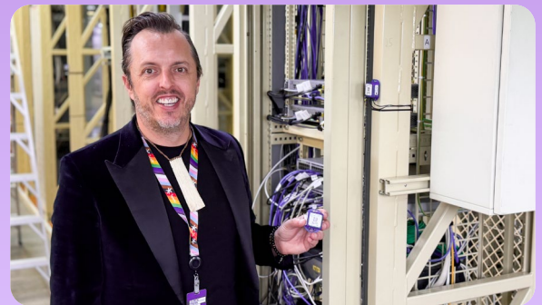
Spark's Autonomous Network Lead, Ulrich Frerk demonstrates a Packet Power sensor which enables real-time power monitoring at the Remuera Exchange.
