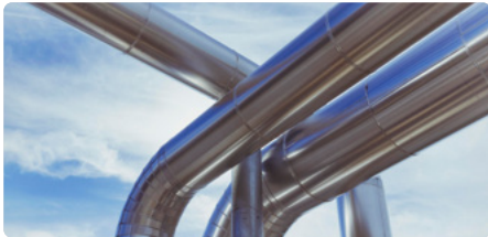
Completed Ngā Tamariki Geothermal Station expansion.
