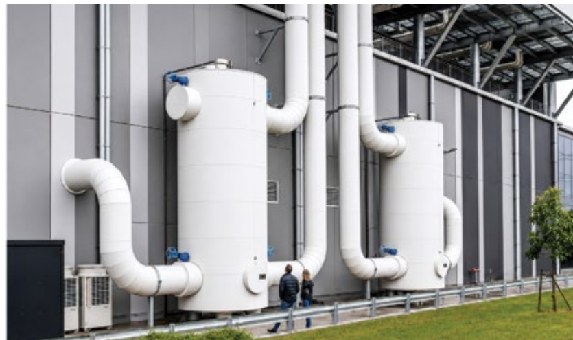
CDC's closed-loop liquid cooling enables near-zero ongoing water consumption for primary cooling.
