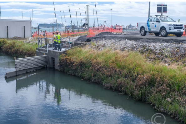
Sulphur Point stormwater treatment system
