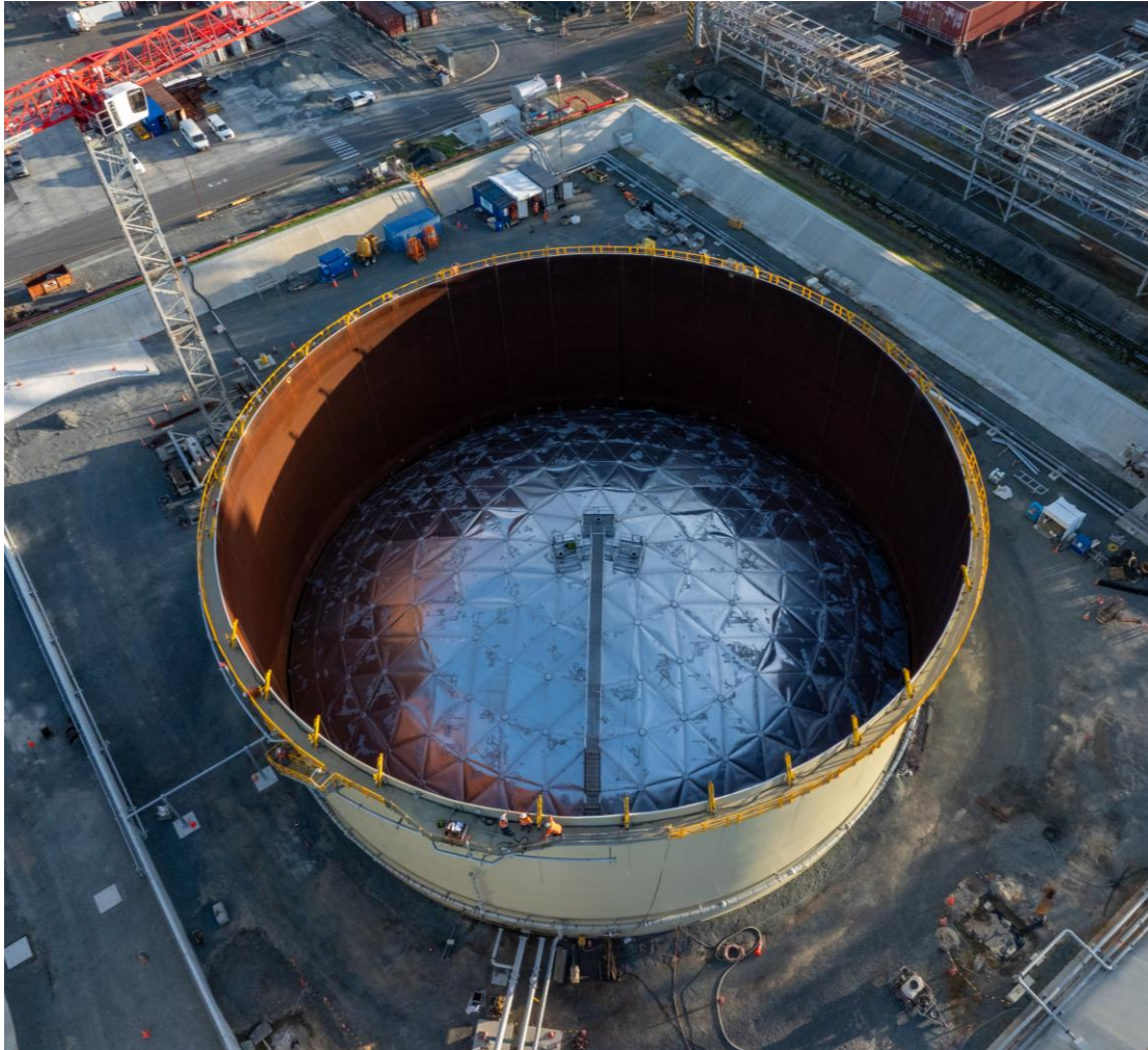
Jet Fuel Storage for Z Energy
